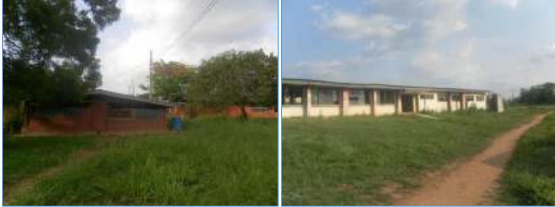
Plate 17: The Poultry and the dilapidated dining hall respectively.
