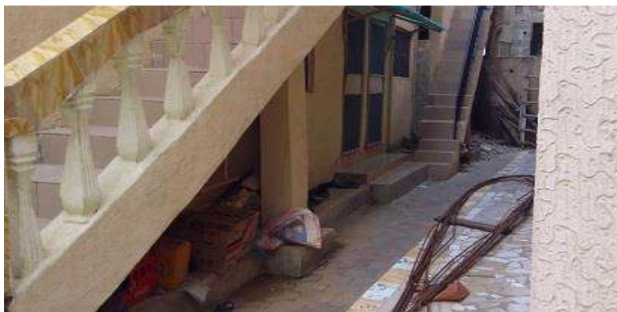
Plate 4.20: State of the setback space between the approach fence and residential building
