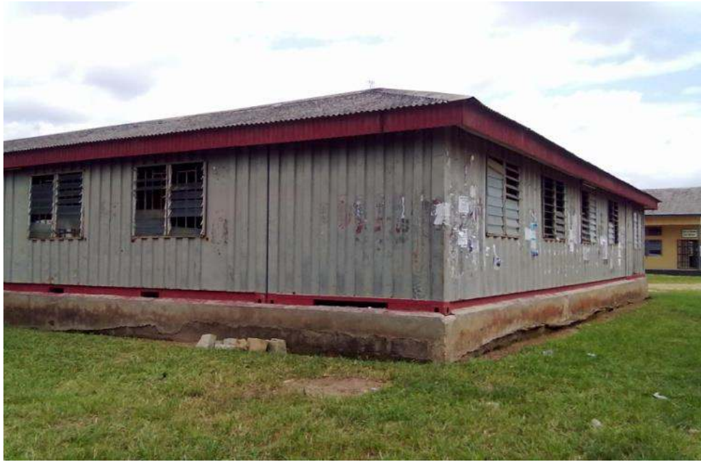
Plate 3.17: A view of the Administrative store of the faculty (UNIUYO) Source: Researcher's Field Work (2015)
