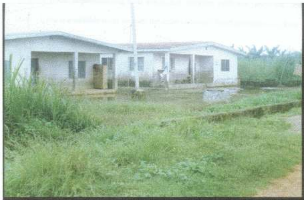
Plate 3: Open gutter not properly inter connected to be functional
