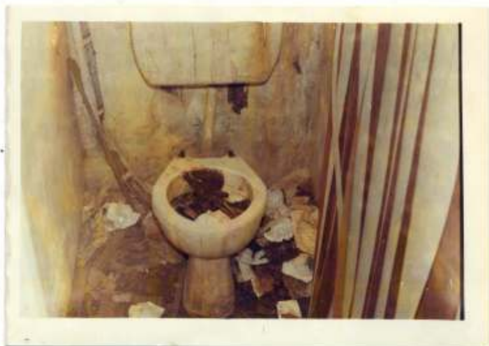
Plate 4.3. A Typical toilet around the laboratories and workshops
