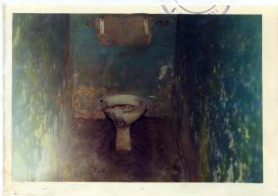
Plate 4.1 A typical hostel toilet, with lavatory pan destroyed and cistern tank removed.
