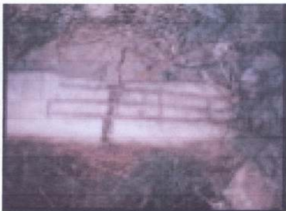
Plate 4.2: In-adequate Cover and large spacing of reinforcement
