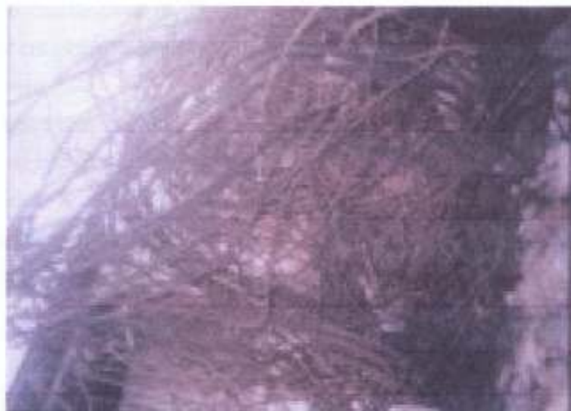
Plate 4.1: Poor Concrete Mix
