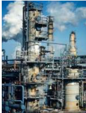
Plate 2: Power Generating Plant
